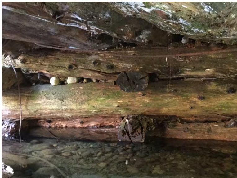
Top face log horizontally cracked
